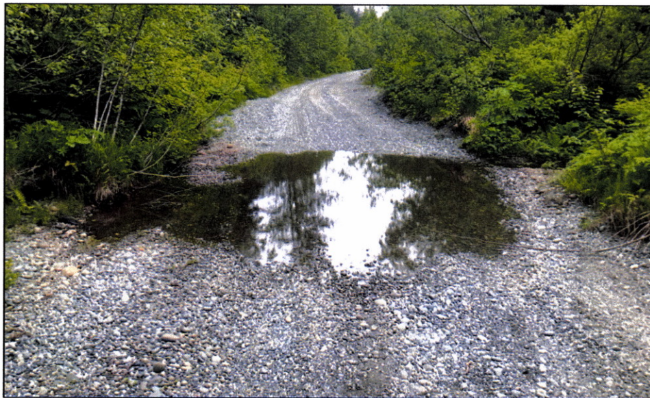
Figure 4.—Water crossing the road at waypoint 266.
