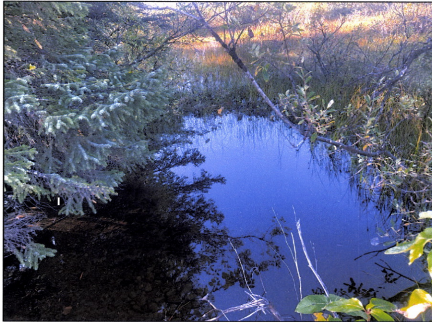
Figure 2. —Water ponded downstream of the culvert.
