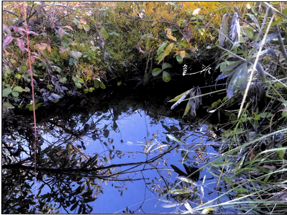
Figure 2. —Water ponded downstream of the culvert.
