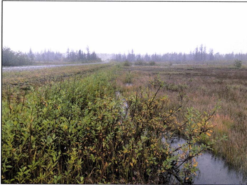
Figure 2. –Diffuse channel looking downstream along the road.
