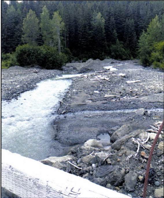
Figure 3.—Berm piles upstream of Carson Creek bridge.
