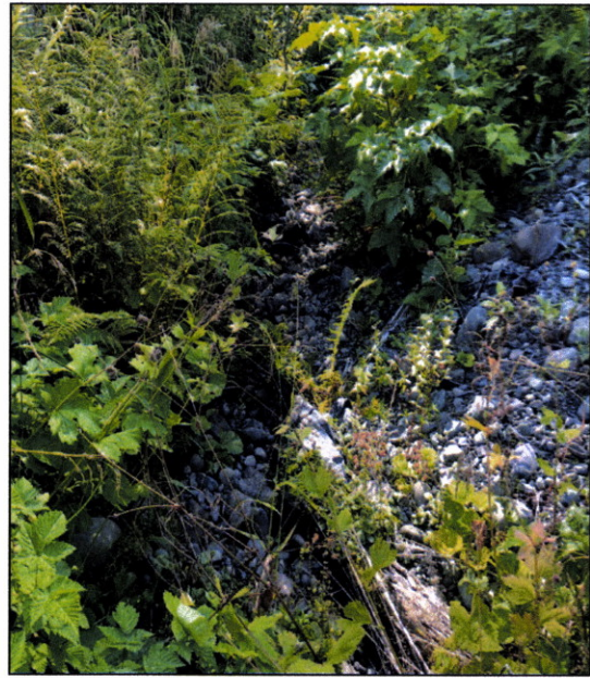
Figure 2.—Debris erosion and dry channel at waypoint 1152.
