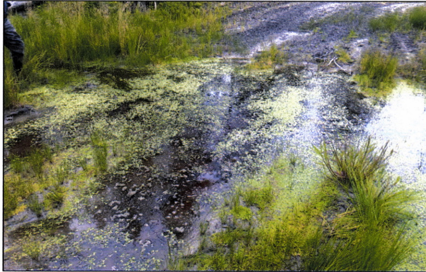
Figure 2. —Ponded water crossing the road at waypoint 760.
