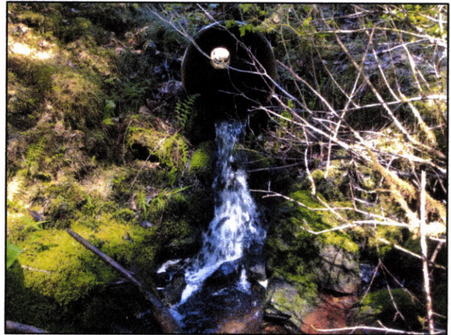
Figure 3.—Perched culvert at waypoint 107.
