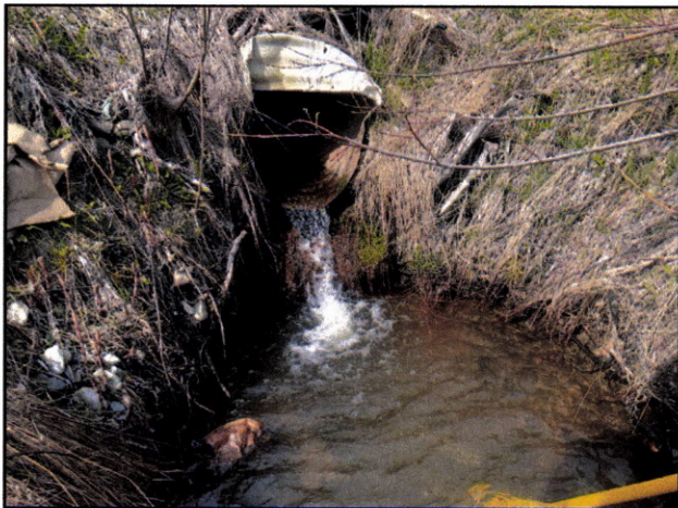
Figure 2.—Perched culvert at waypoint 1425.
