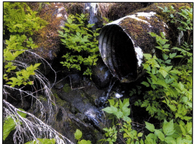
Figure 3.—Perched pipe outlet at waypoint 68.
