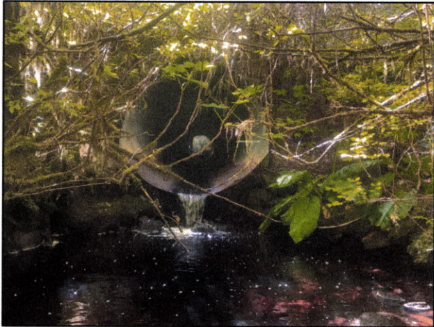
Figure 2.—Perched culvert at waypoint 1000.
