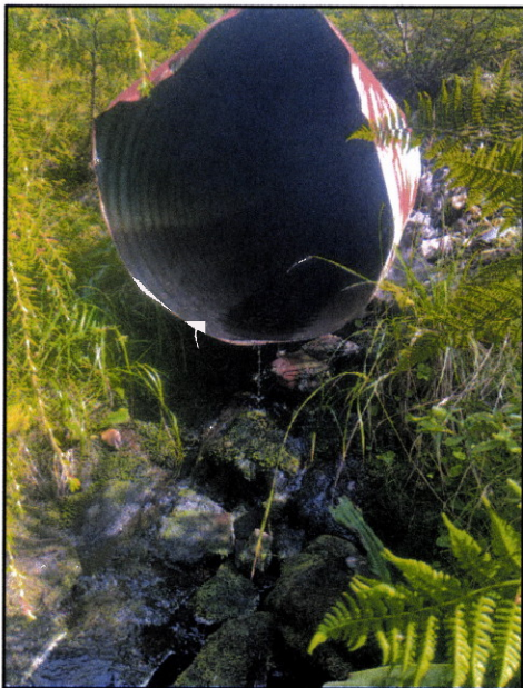
Figure 2.—Perched culvert at waypoint 1007.
