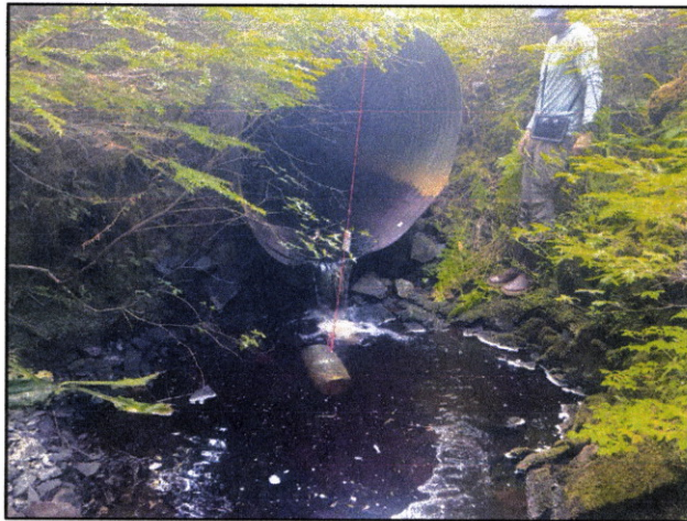
Figure 2.—Channel flowing through perched culvert at 1008.
