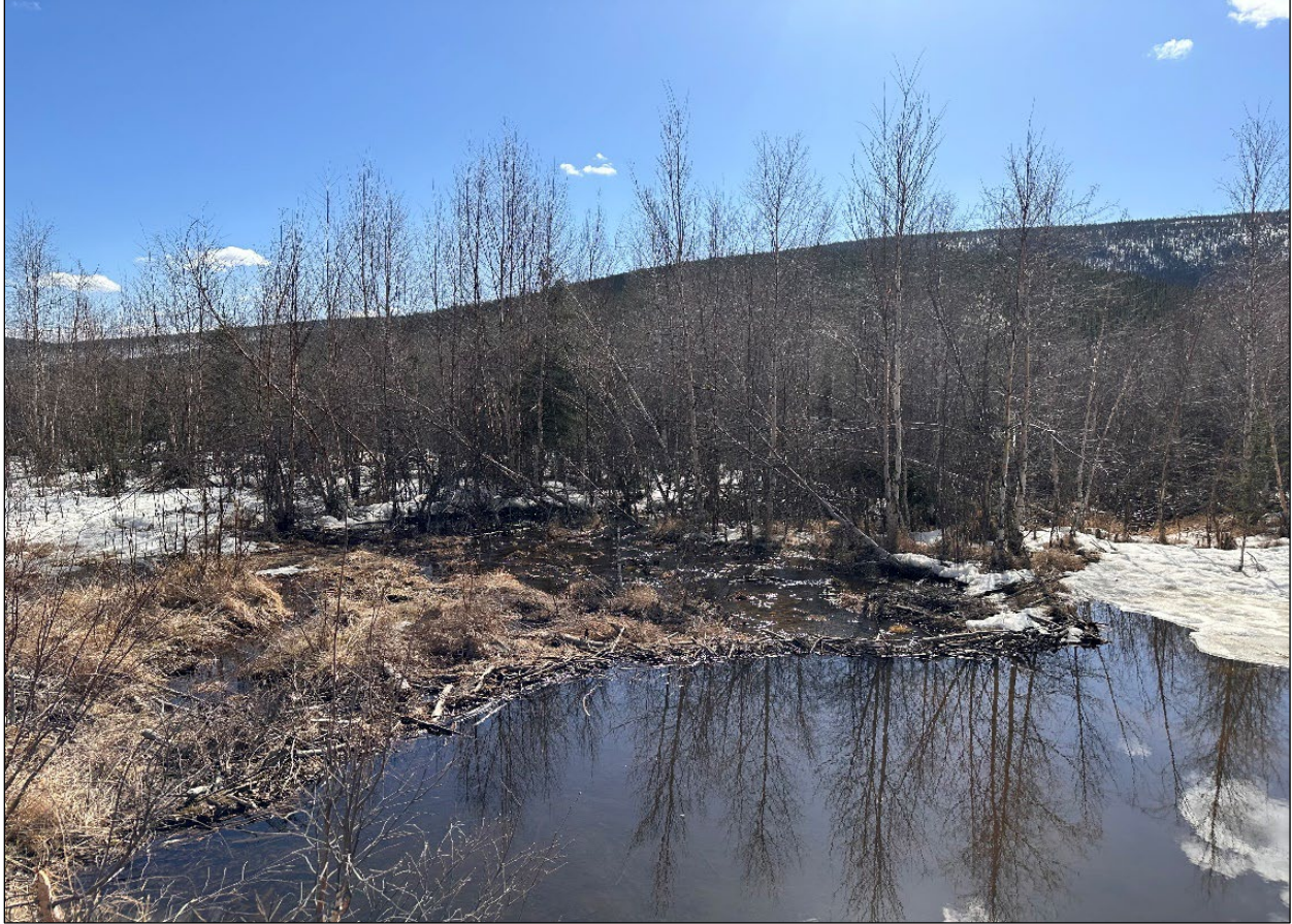
Figure 40. RO water exiting Pond AB and into Fish Creek, bypassing the blocked outlet culverts, April 2024.
