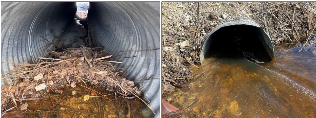
Figure 39. Pond AB culverts were blocked during fall of 2023 and cleared by ADF&G staff in April 2024, returning water flow to the RO Channel.
